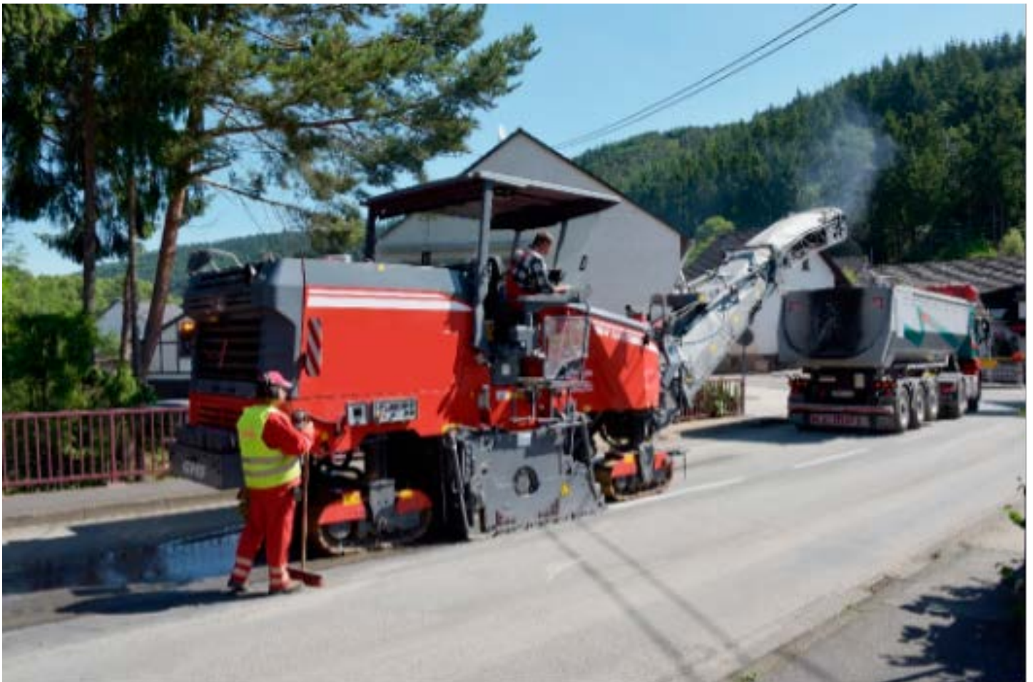
Figure 4. Milling of existing asphalt pavement to recover the material and re-use it in the construction and maintenance of new roads
